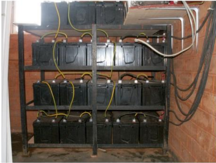
Figure 15.9: A battery bank of 3600 Ah, currents reach levels of 45 A during charging
