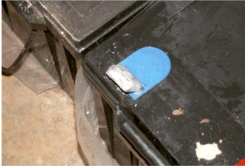
Figure 14.2: A 200 Ah lead-acid battery. The negative terminal was broken due to weight on the terminals during transportation.
