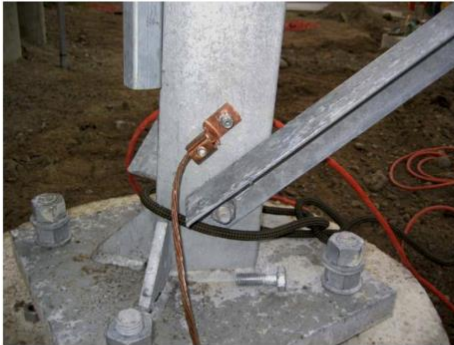
Figure 11.3: A tower with a heavy copper grounding wire.
