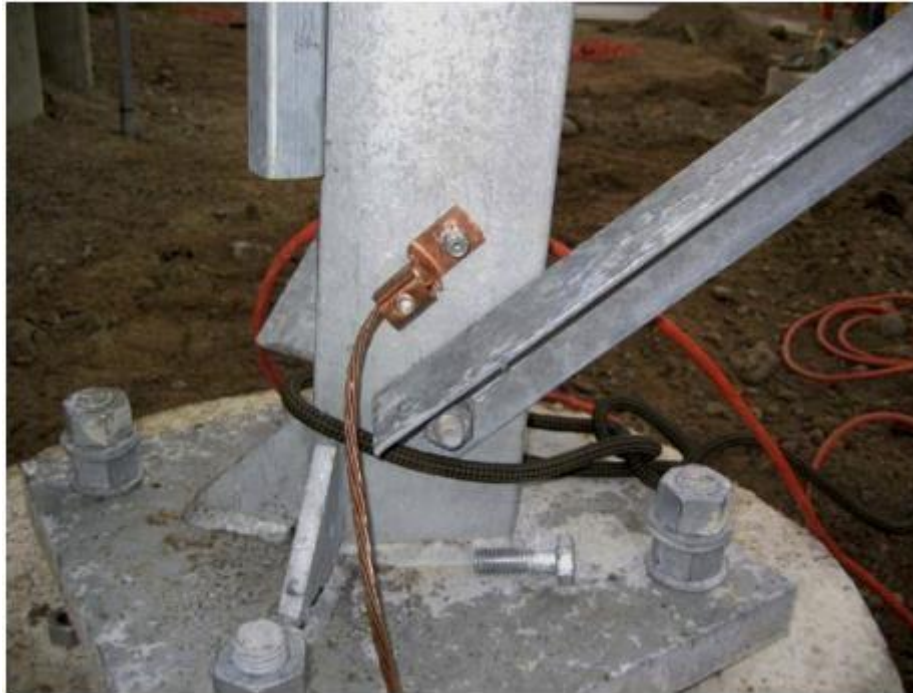
Figure 11.3: A tower with a heavy copper grounding wire.
