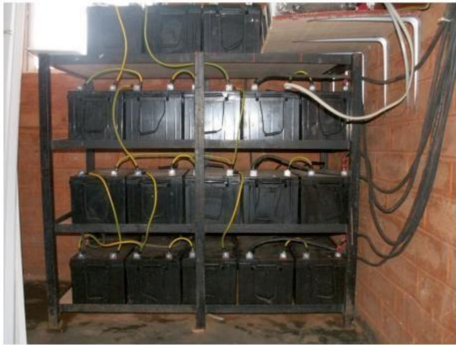
Figure 15.9: A battery bank of 3600 Ah, currents reach levels of 45 A during charging
