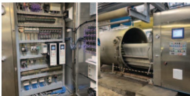
The 5.5 kW ABB industrial drive ensures a uniform dyeing or bleaching process by maintaining a constant tension in the wound fabric as the diameter of the reel changes.
