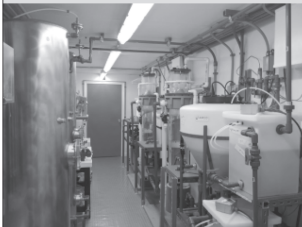
The PFAS compounds extracted from the ground are destroyed using an ultraviolet light technology inside this trailer. (Photo courtesy of EnChem Engineering Inc)
